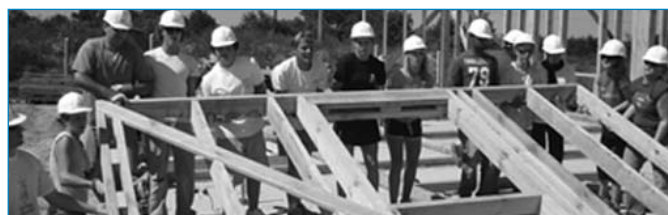
Raising a wall on the Habitat for Humanity site in Csurgó, Hungary.
